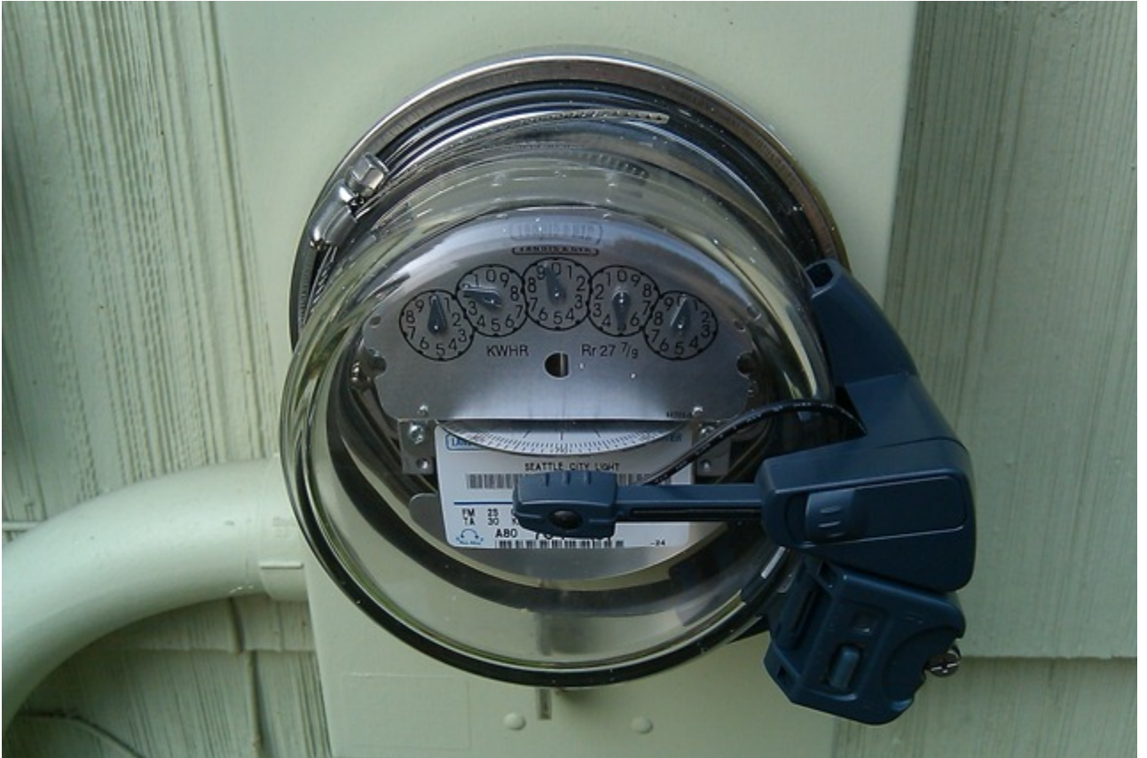
PowerCost Monitor sensor attached to my house's power meter
