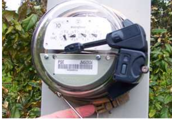
Outdoor device attached to PSE meter face
